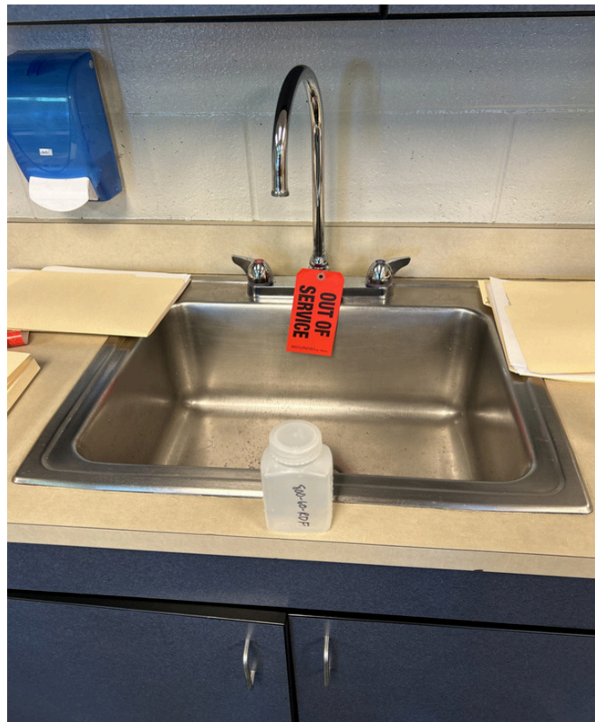
6/27/2024 - 800-60 - Discovery Middle School- Classroom 205 - 004265-Room 205-Right Sink
