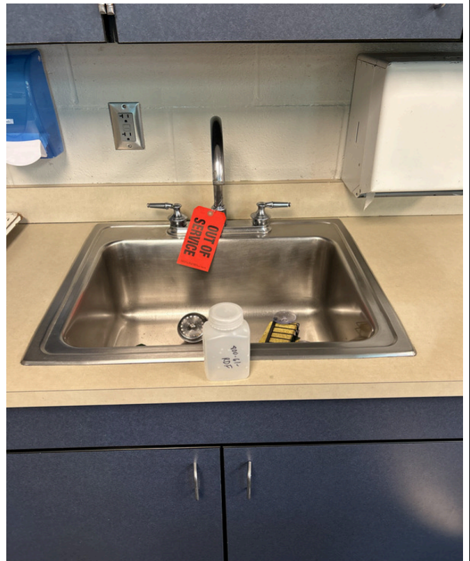
6/27/2024 - 800-61 - Discovery Middle School- Classroom 205 - 004266-Room 205-Left Sink
