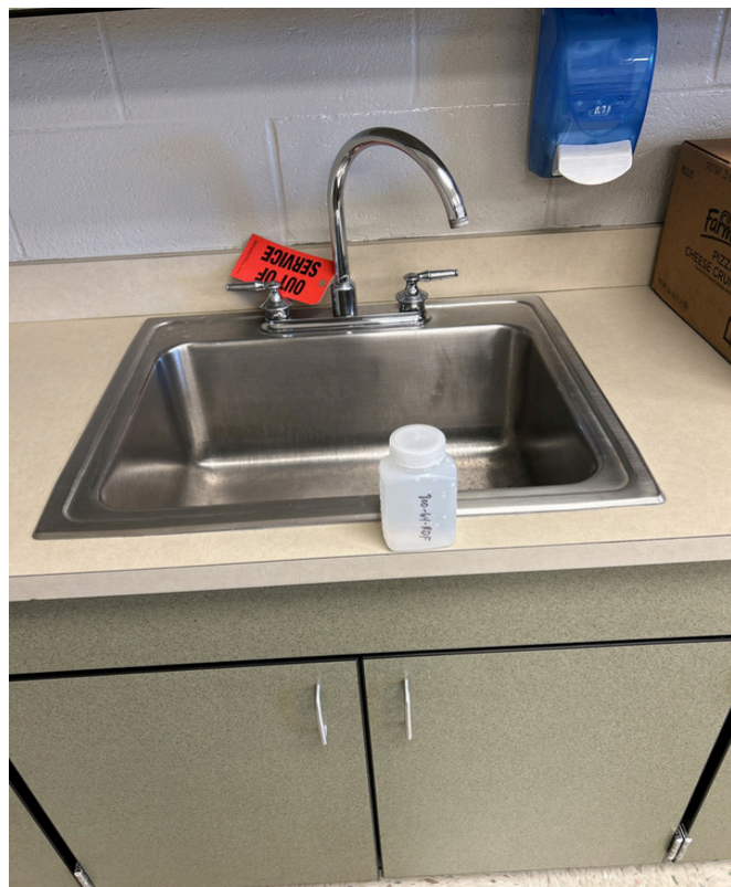
6/27/2024 - 800-64 - Discovery Middle School- Classroom 207 - 004262-Room 207-West Wall- Left Sink
