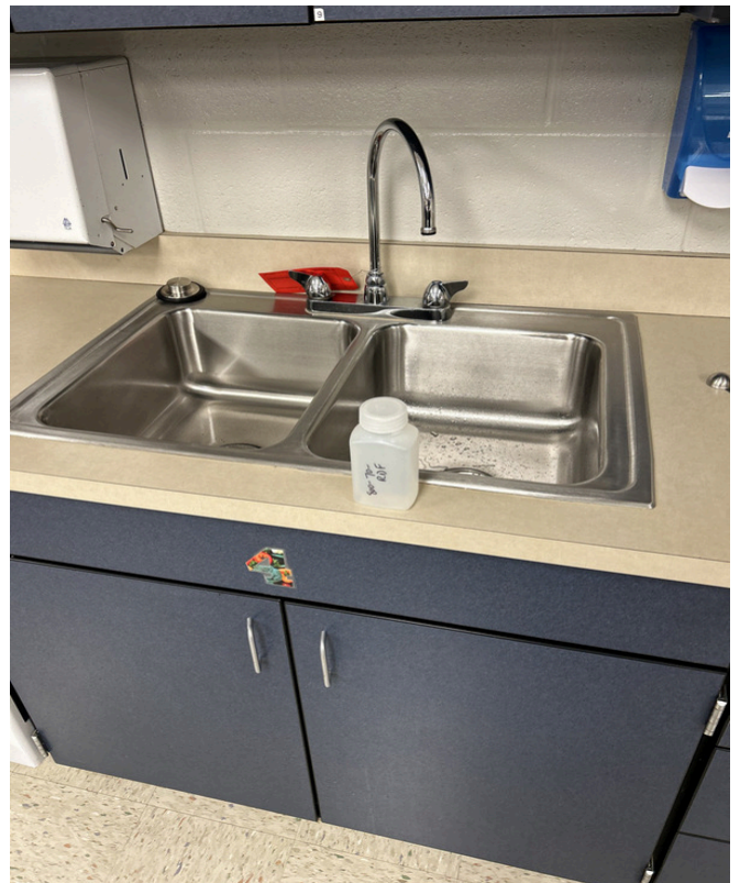
6/27/2024 - 800-70 - Discovery Middle School- Classroom 206 - 004256-Room 206-Kitchen 4
