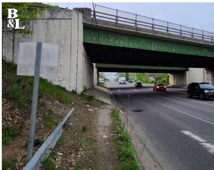
Figure 18 - Worn Pedestrian Foot Path on Payne Road
