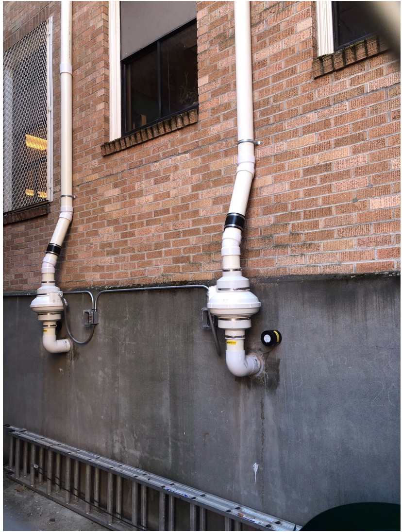
System #2 & 3 mitigation fans are located in the western fenced courtyard. Two AMG Fury model fans were used due to the porous soil beneath the concrete slab in the crawlspace below rooms 152, 163 and 164. Each fan has an exterior rated pressure gauge
