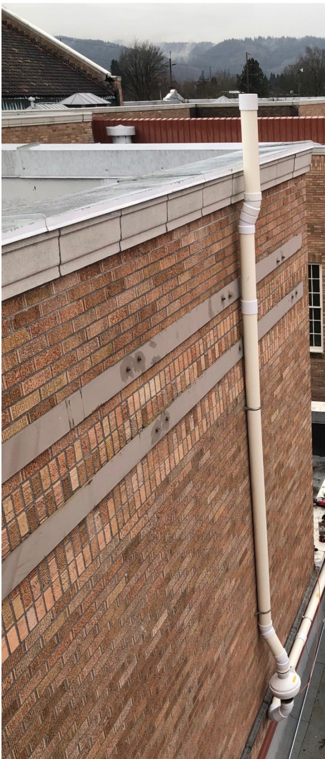
System #1 mitigation fan is located on the eastern roof of the building. A single AMG Eagle model fan was used due to the less porous soil beneath the concrete slab of room 19.
