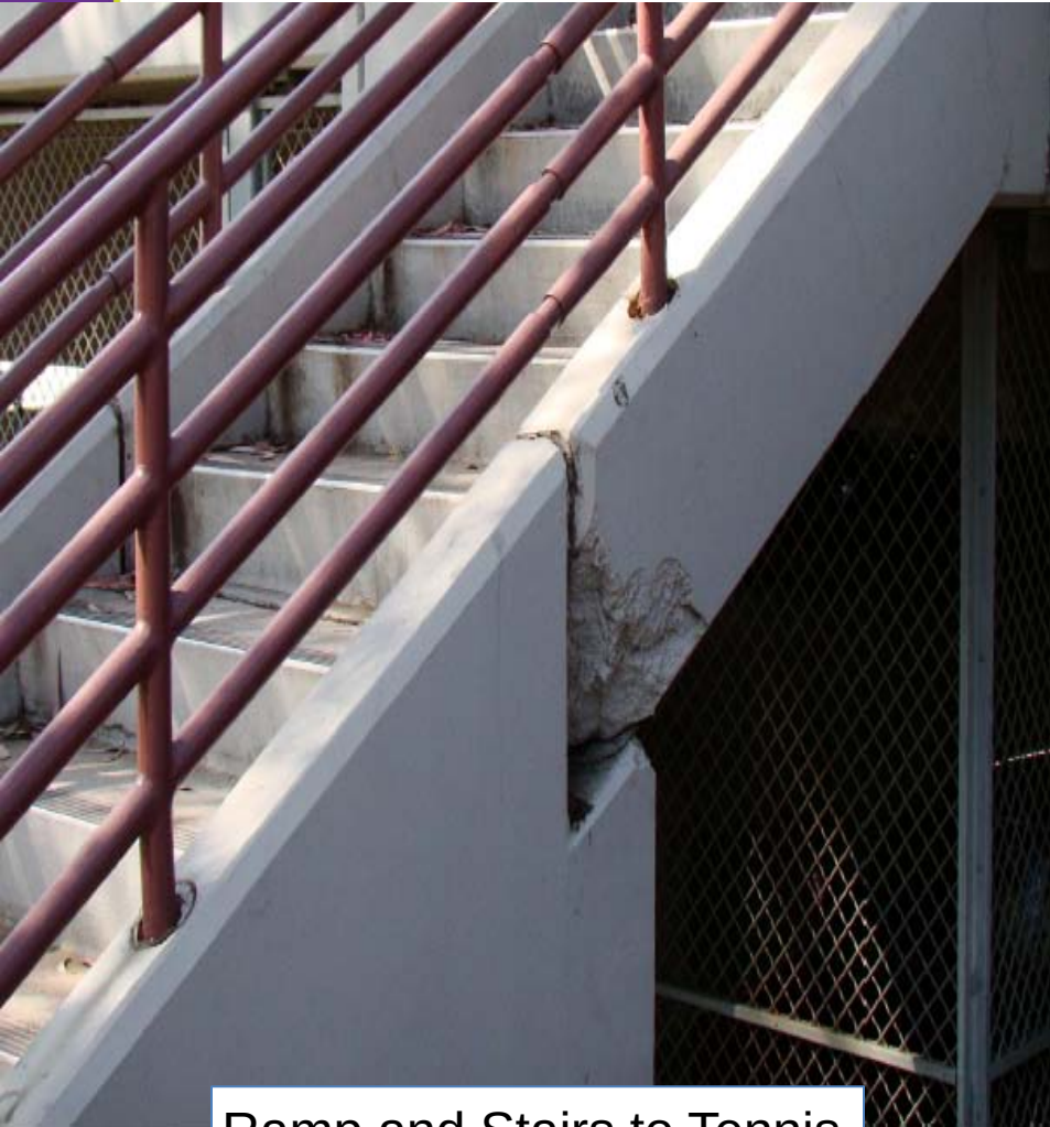
Ramp and Stairs to Tennis Courts are Cracked
