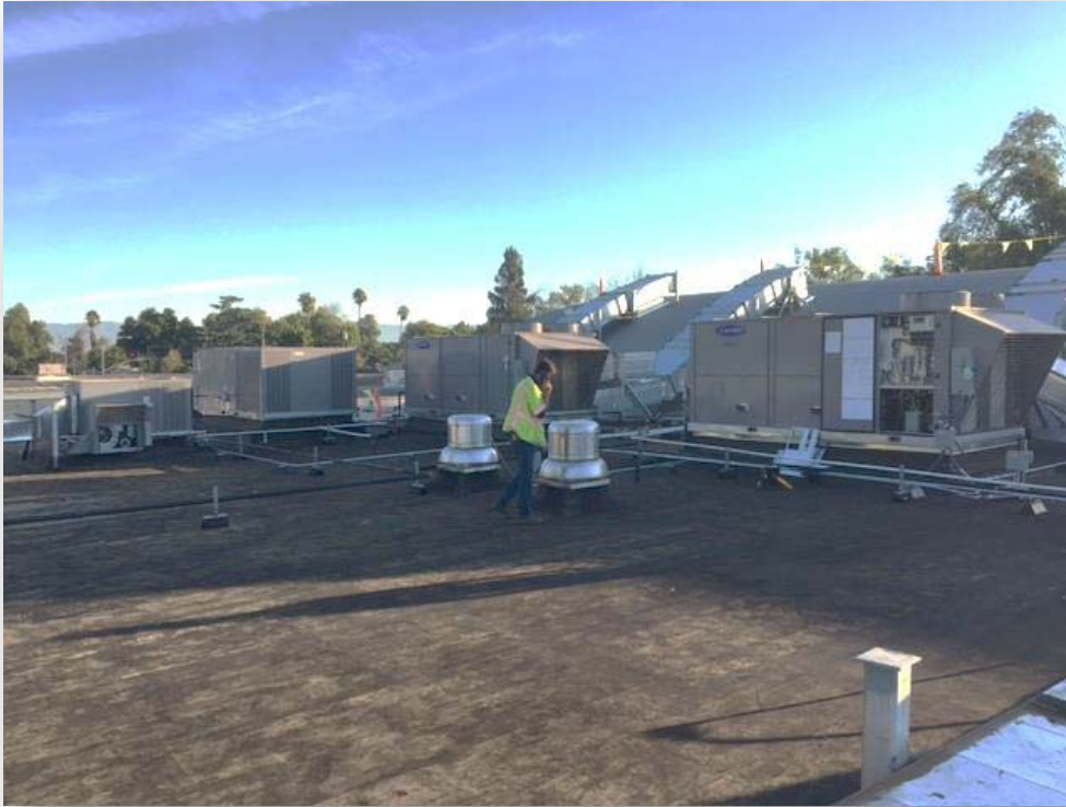
HVAC start up on Gymnasium roof
