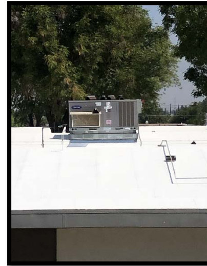
New HVAC Units
