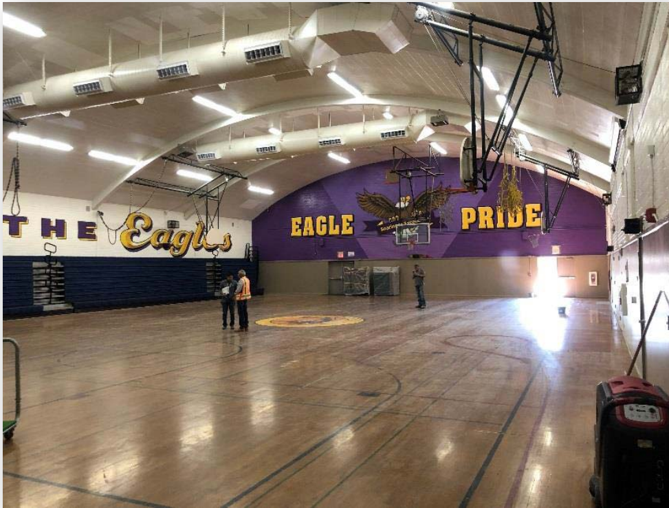
HVAC start up on Gymnasium roof
