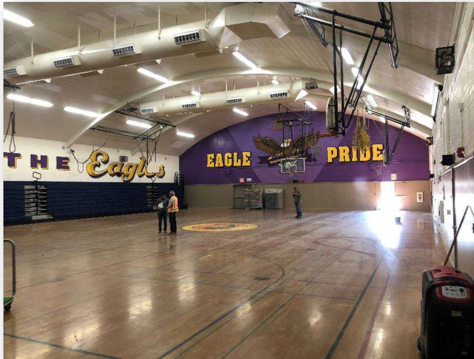
HVAC start up on Gymnasium roof
