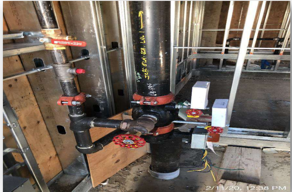
New fire riser installed and tested in the new kindergarten building
