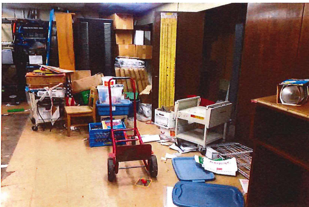
Will Rogers – Electrical Room - Before
