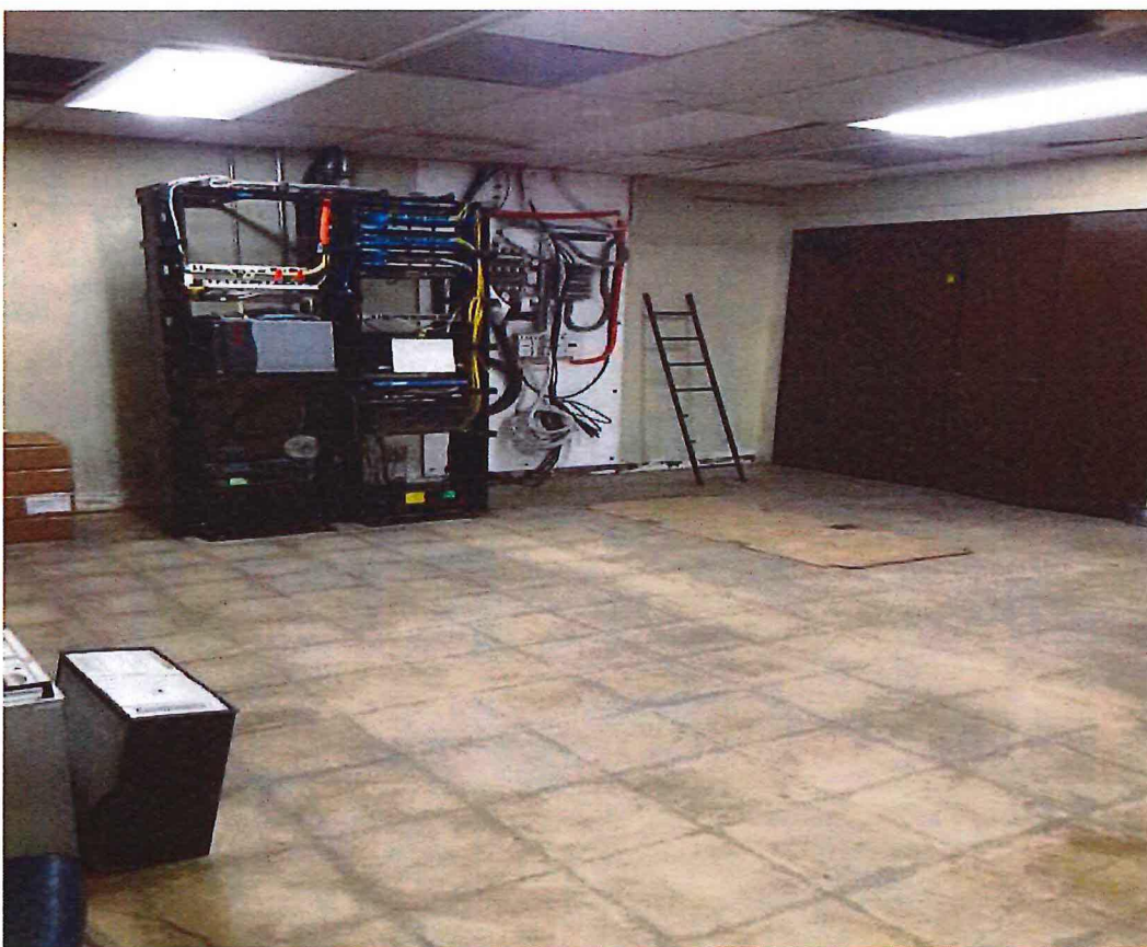
Will Rogers – Electrical Room - After
