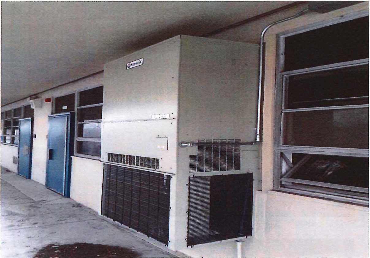
Vista HS – New Energy Efficient HVAC System
