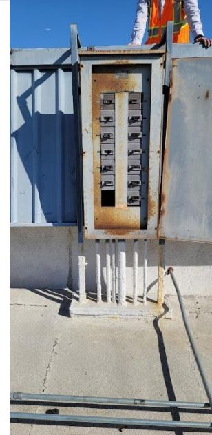
Will Rogers ES HVAC Replacement Project – Existing Electrical Panels will be Replaced
