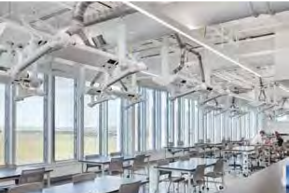
OVERHEAD DISTRIBUTION SERVICE CARRIER
