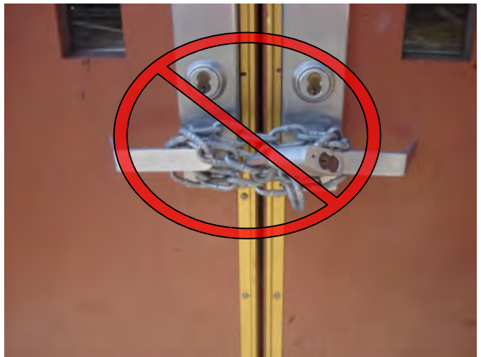
Building exit doors can never be chained or padlocked, either from the inside or the outside.
