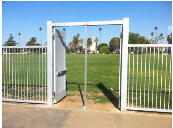
Gates between the buildings and the Safe Dispersal Area must have panic hardware and can never be chained or padlocked, day or night.
