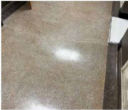
Crack in hallway
