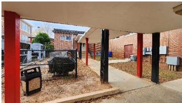
Building 5030 Stairs 1: Located outside of the cafeteria and leads to the covered walkway.
