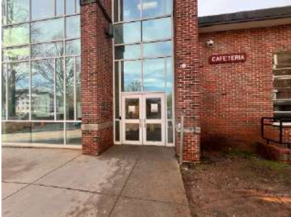
Building 5040 Door 2 and 3: Located on the front façade of the building under a glass walkway.
