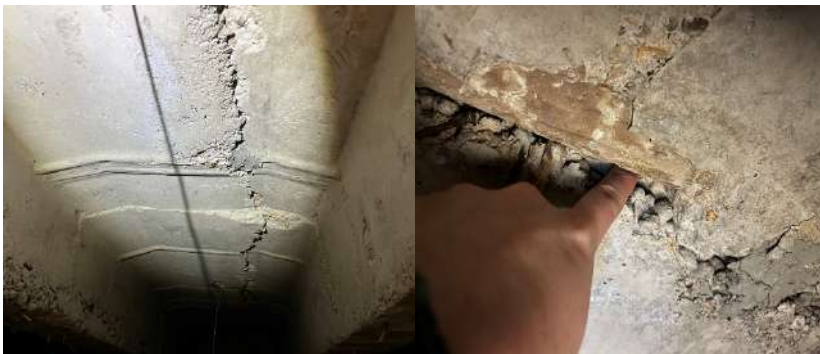
Spalling in floor joist
