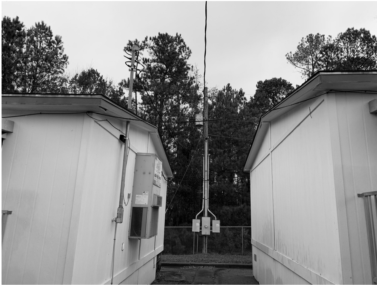
DOMINION ENERGY TRANSFORMER POLE
