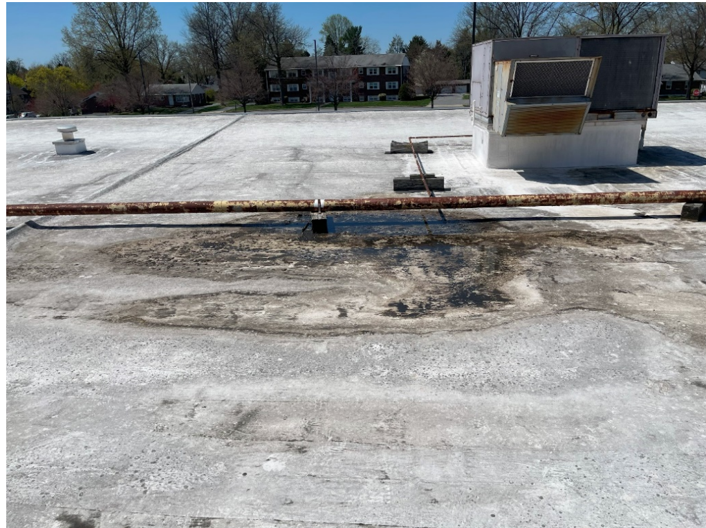
Gas piping, HVAC units, Ponding
