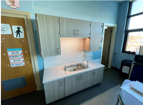
WBS - Classroom backsplash panels replaced from manufacturing defect
