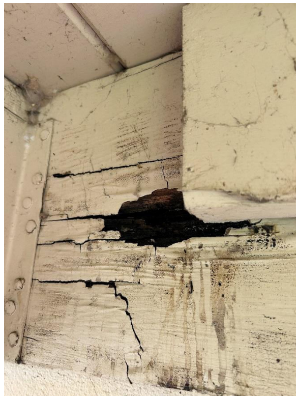
Wood coating in poor condition
