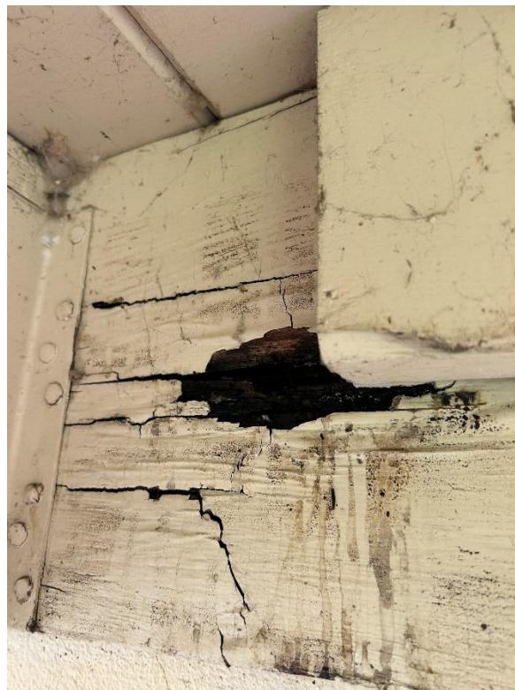
Wood coating in poor condition
