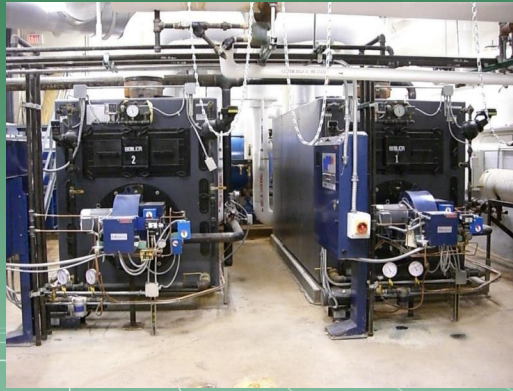
NEW BOILERS and BURNERS
