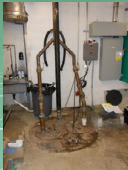
EXISTING OLDER BOILERS AND PUMP SYSTEMS
