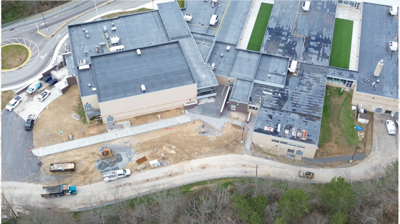
Eastern view of school. Bus drop-off sidewalk is in, and entrance walkways are being formed for concrete
