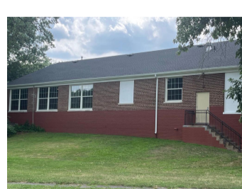
Field House Phase I is complete! Our Bulldogs will have access to it this Fall. Phase II starts next spring!
