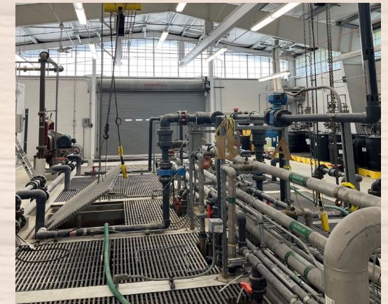
WASTEWATER TREATMENT FACILITY – 4,300 sq. ft (2009)
