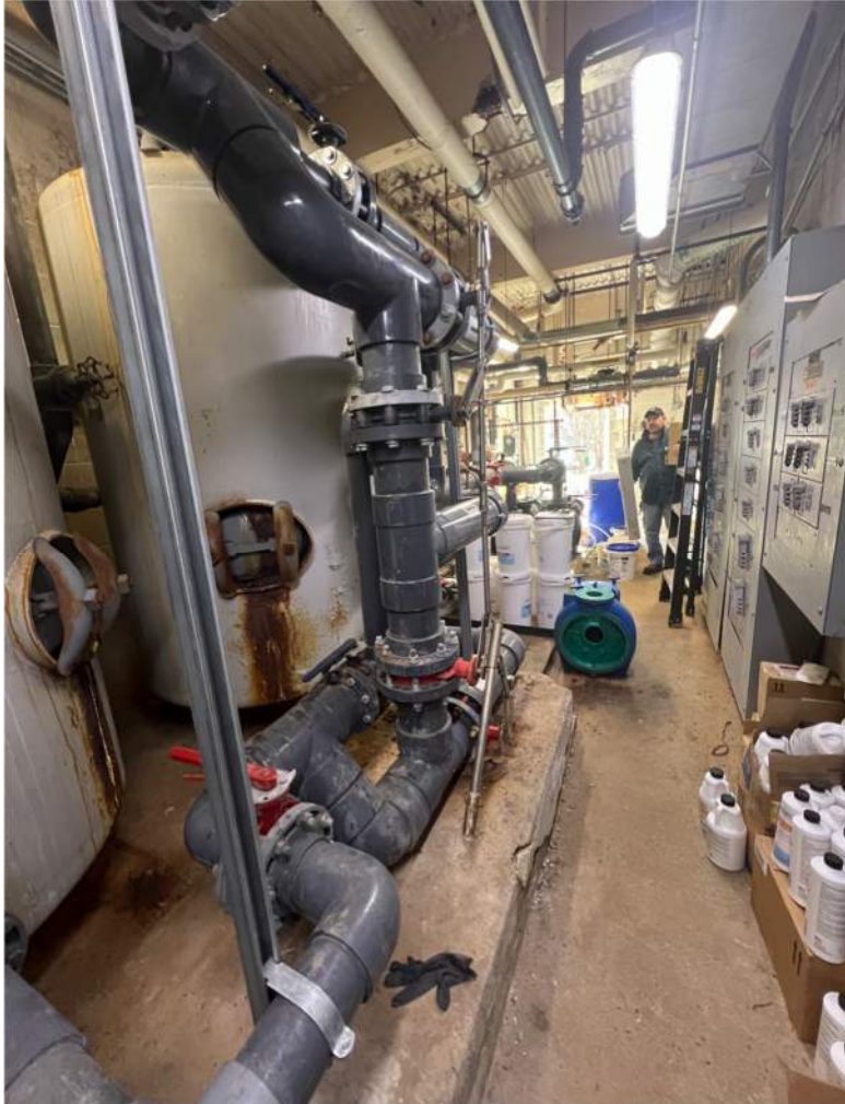
Photo 28: The proximity of the filters to the electrical panels is problematic, as is the storage of chemicals in close proximity to the electrical equipment.
