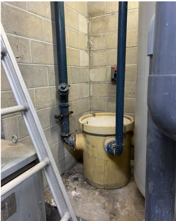
Photo 33: There is an acid neutralization system located behind the filters, that serves laboratories in another area of the building. Its condition and function was not reviewed as part of this report, but in a planned renovation it needs to be accounted for in the space planning.
