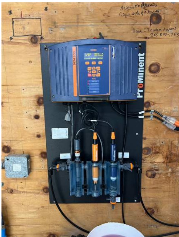
Photo 31: Chemicals are automatically monitored and fed through a chemical controller. The Prominent Unit installed at the pool is relatively new and is appropriate for continued use.
