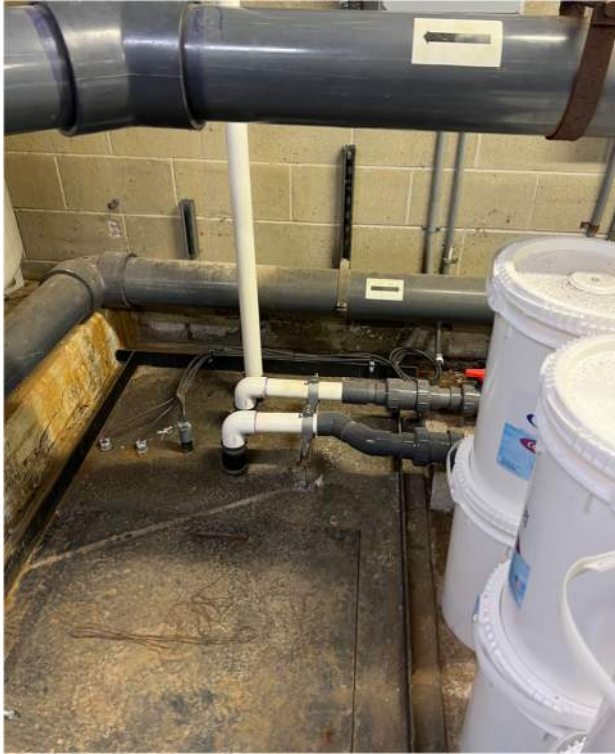
Photo 32: An sewage ejector pit is located in the Filter Room. When renovations are planned, the capacity and location of discharge of this system should be confirmed to determine if it can be used for filter back-wash water, in addition to other sanitary waste it serves.
