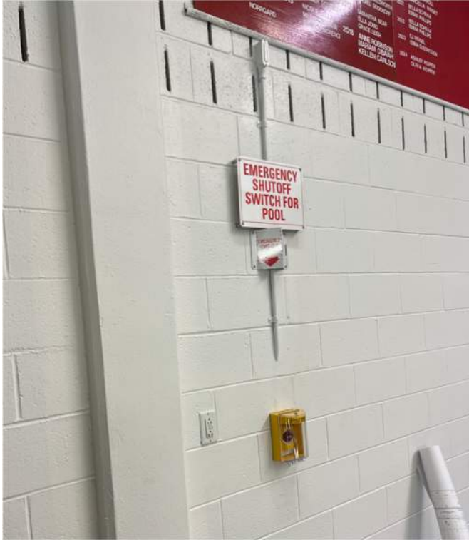
Photo 11: To mitigate risk resulting from the main drain configuration, Greenwich Public Schools installed an emergency shut-off switch to shut down the pumps in the case of an emergency, releasing suction at the drains. Our understanding is that the shut-off plunger is staffed by a trained individual at all times when the pool is occupied.
