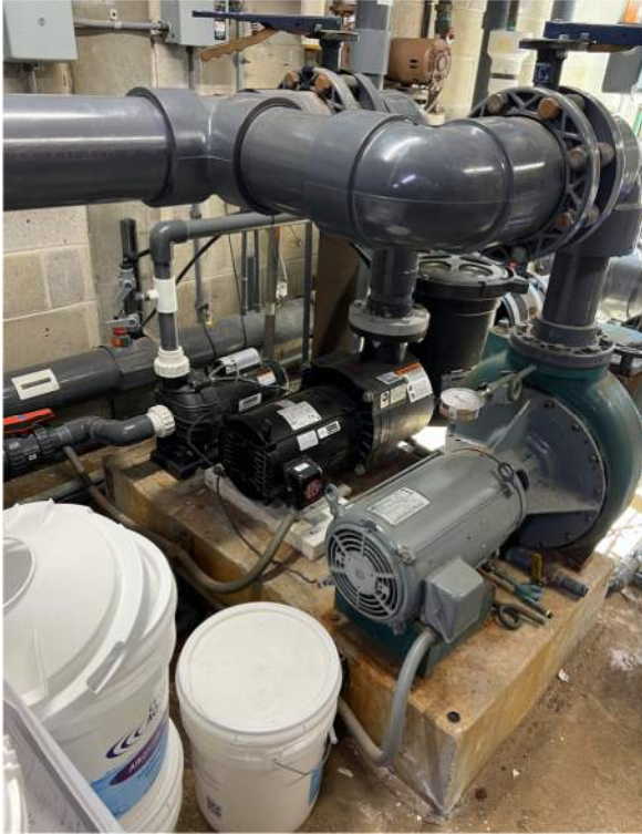
Photo 26: Dual recirculation pumps draw water from the surge tanks and send it to the filters. Pumps run in tandem to deliver 635 GPM through the system.
