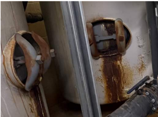
Photo 29: Significant rust at the filter manways, indicates leaks and likely weakening of the pressure vessel's steel shell. It has been reported that filter media is discharged to the pool during backwash, indicating failed laterals within the filters.
