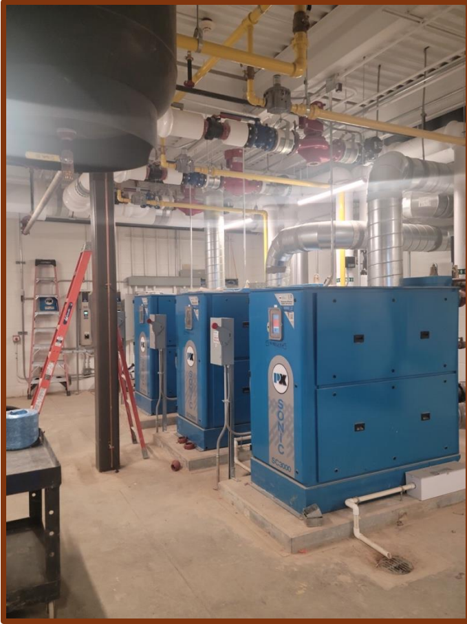
Mechanical Room – HVAC Boilers
