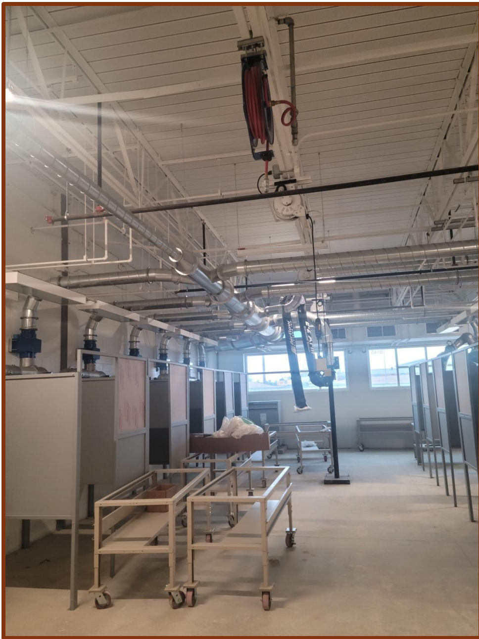
Area B – Ag Mechanical Room
