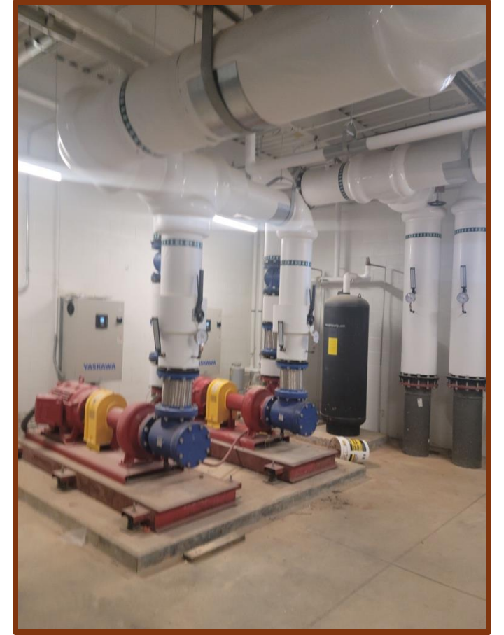
Mechanical Room – HVAC Pumps
