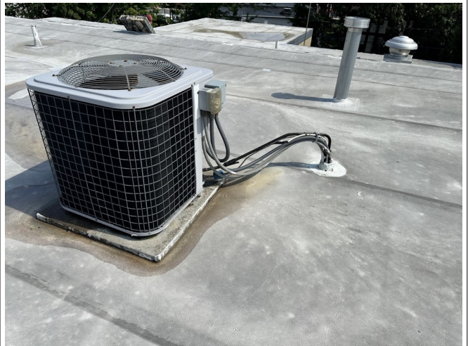
HVAC Pipe Penetration Sealant
