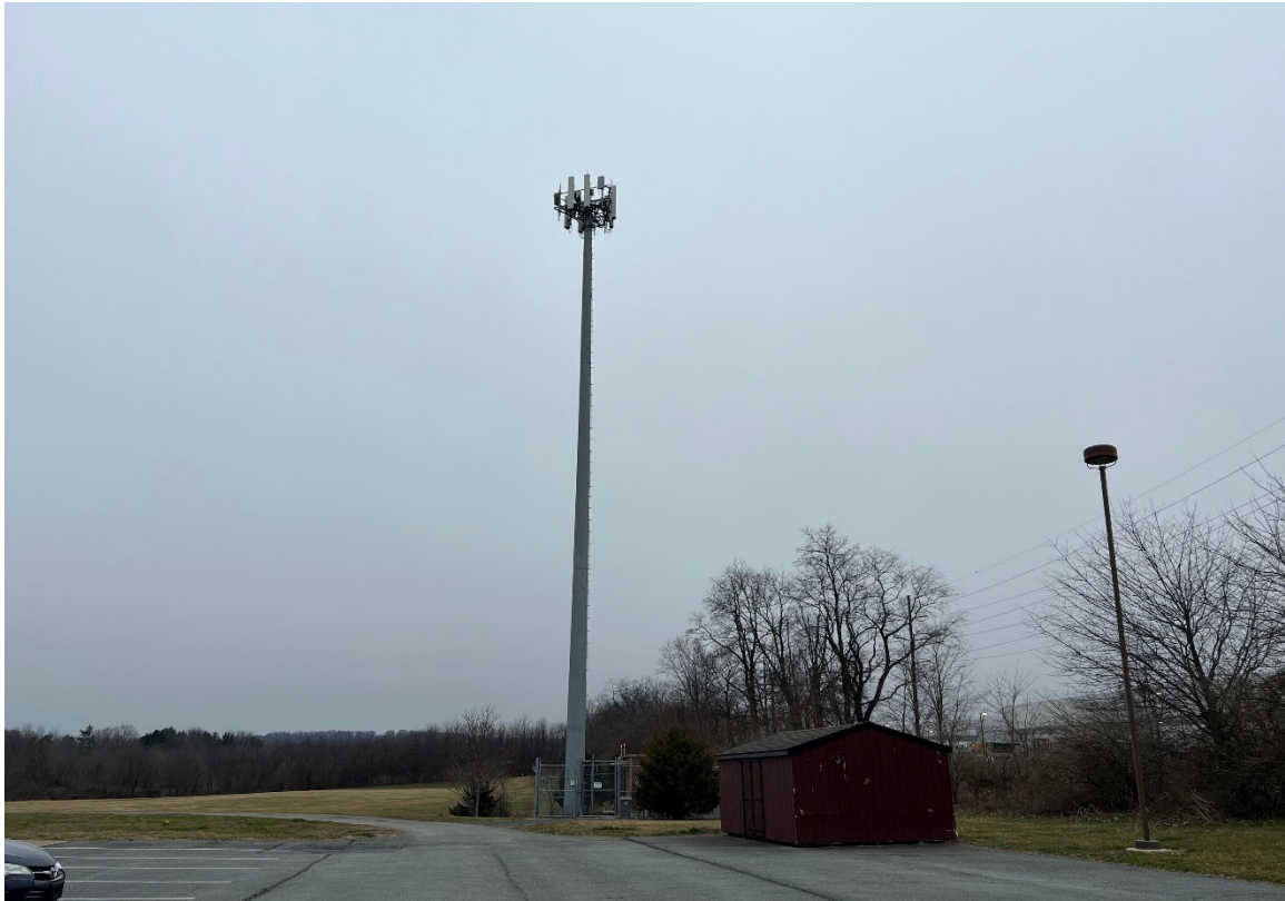
Monopole with Cell Antenna Installation
