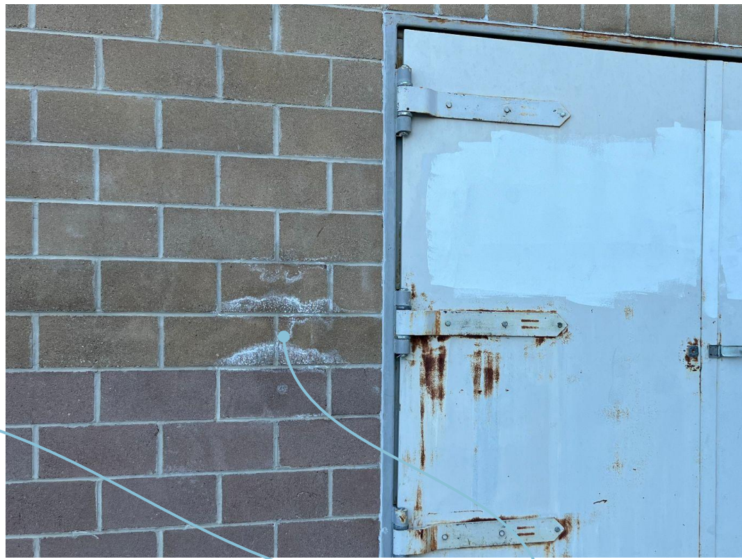
Exterior Walls CMU Block Water damage
