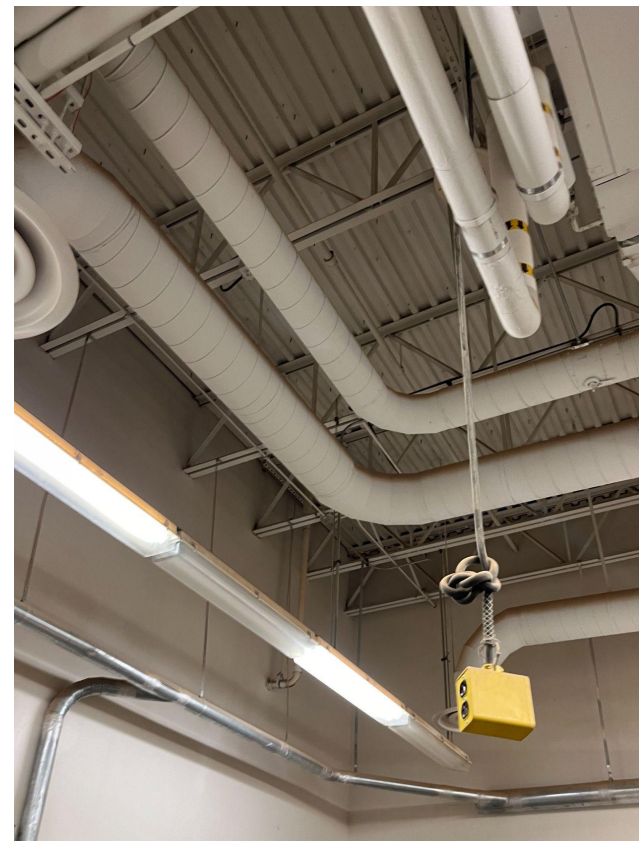
CTE Woodshop exhaust system
