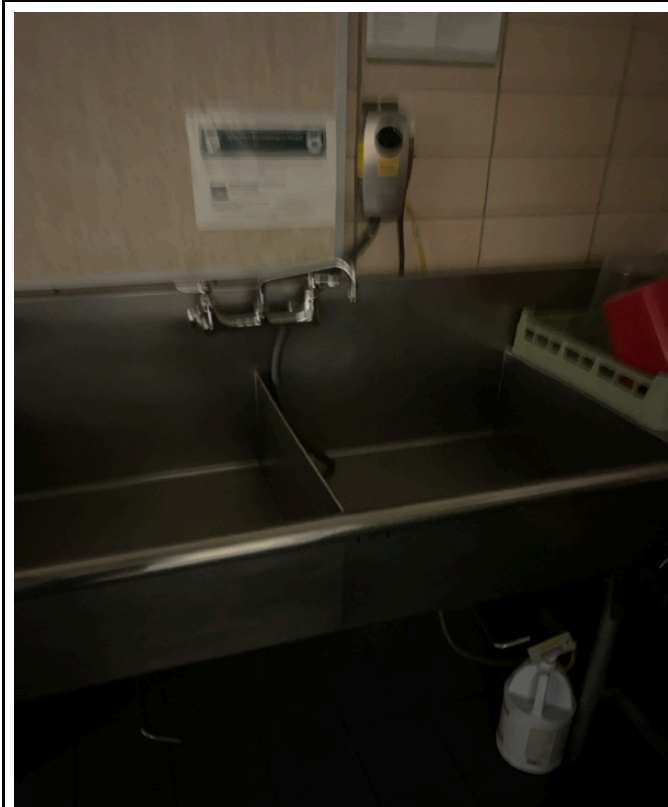
3/28/2024 - 1400-87 - Manor Hill - 001046-Kitchen
