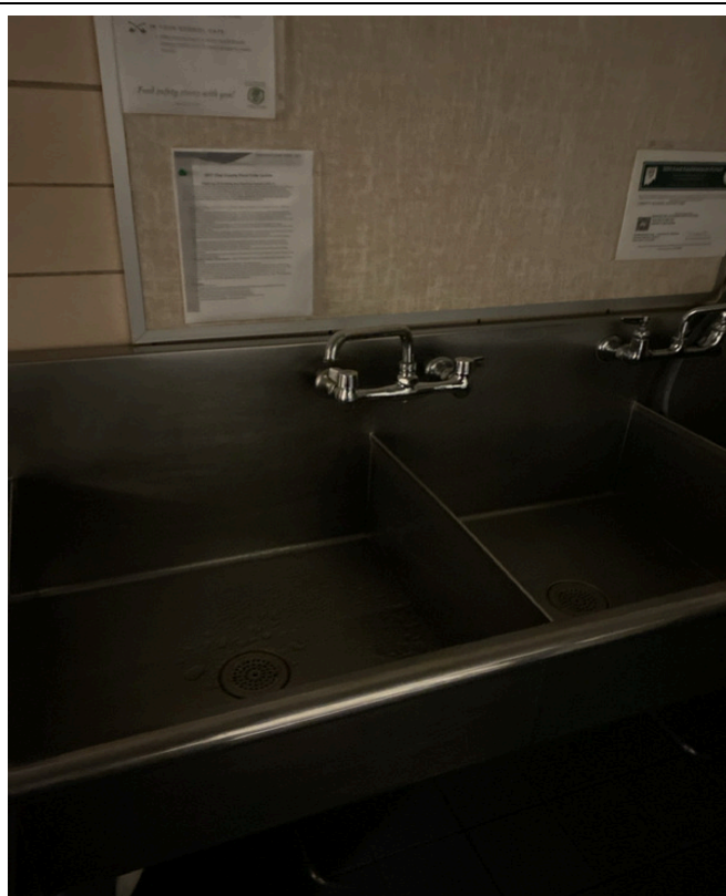
3/28/2024 - 1400-86 - Manor Hill - 001045-Kitchen
