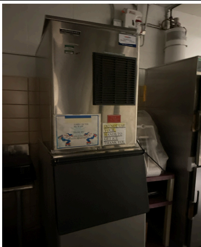
3/28/2024 - 1400-88 - Manor Hill - 001047-Kitchen
