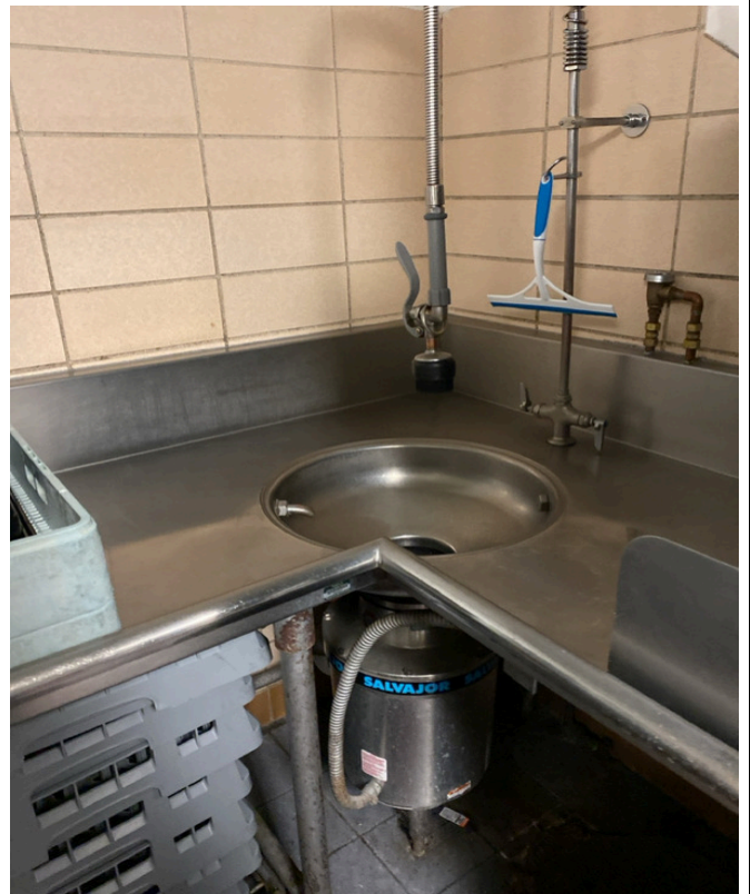
3/28/2024 - 1400-82 - Manor Hill - 004512-Kitchen
