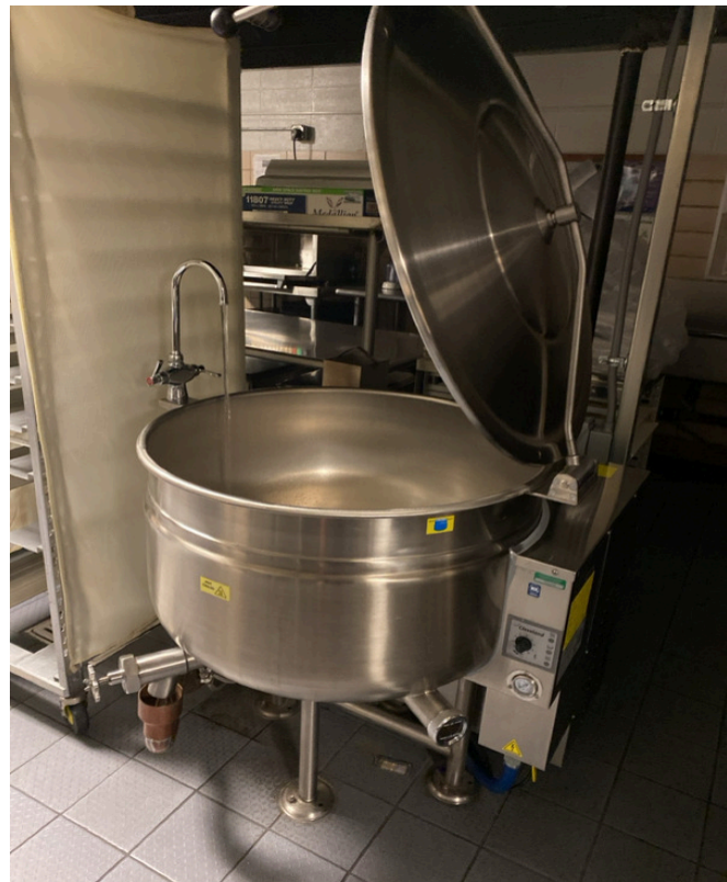
3/28/2024 - 1400-81 - Manor Hill - 000849-Kitchen
