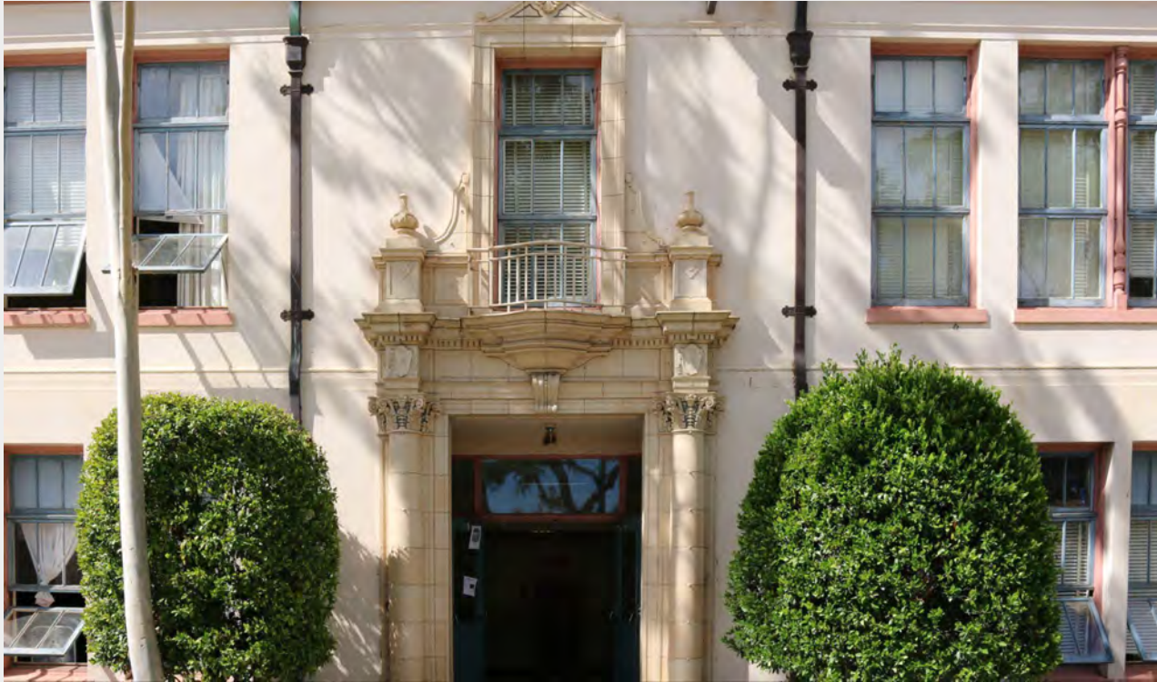
SBHS Windows Rehabilitation (Before)
