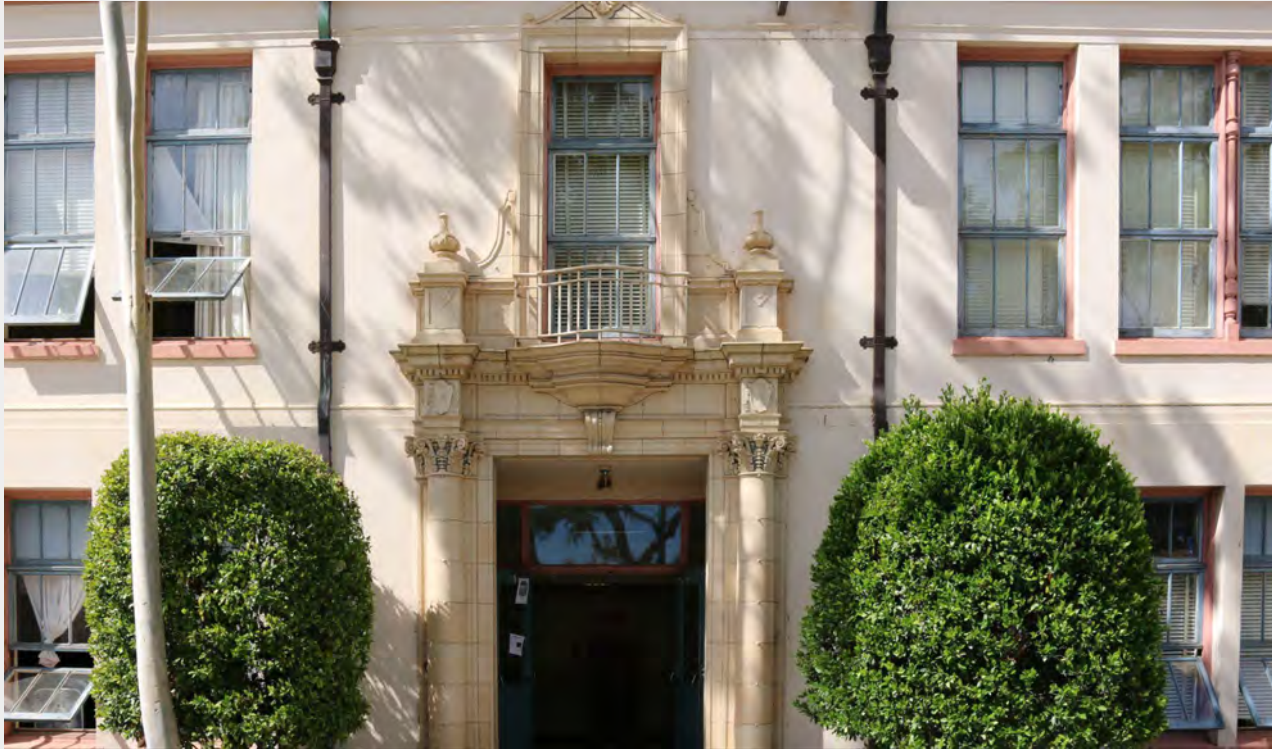
SBHS Windows Rehabilitation (Before)
