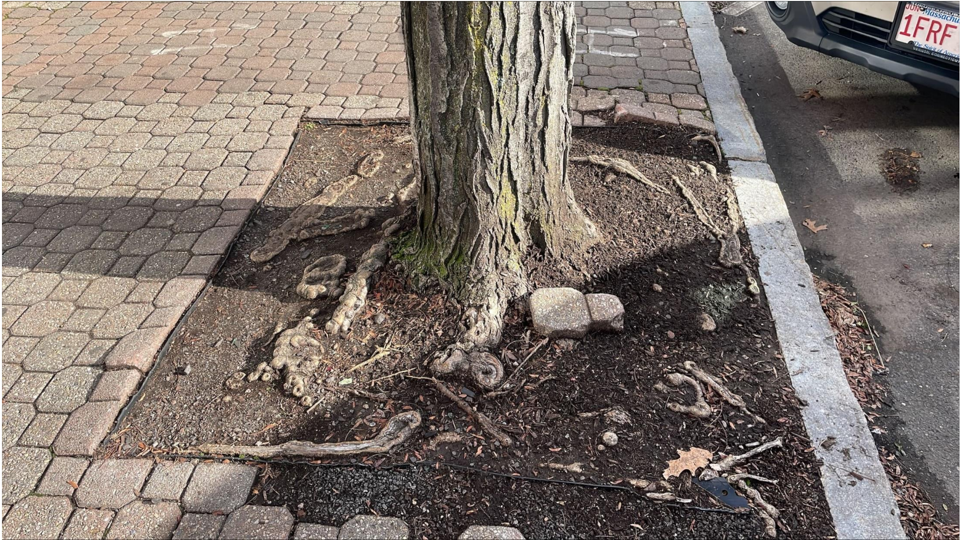
Thornless honey locust # 2, showing girdling roots, damaged roots, and sidewalk damage.
