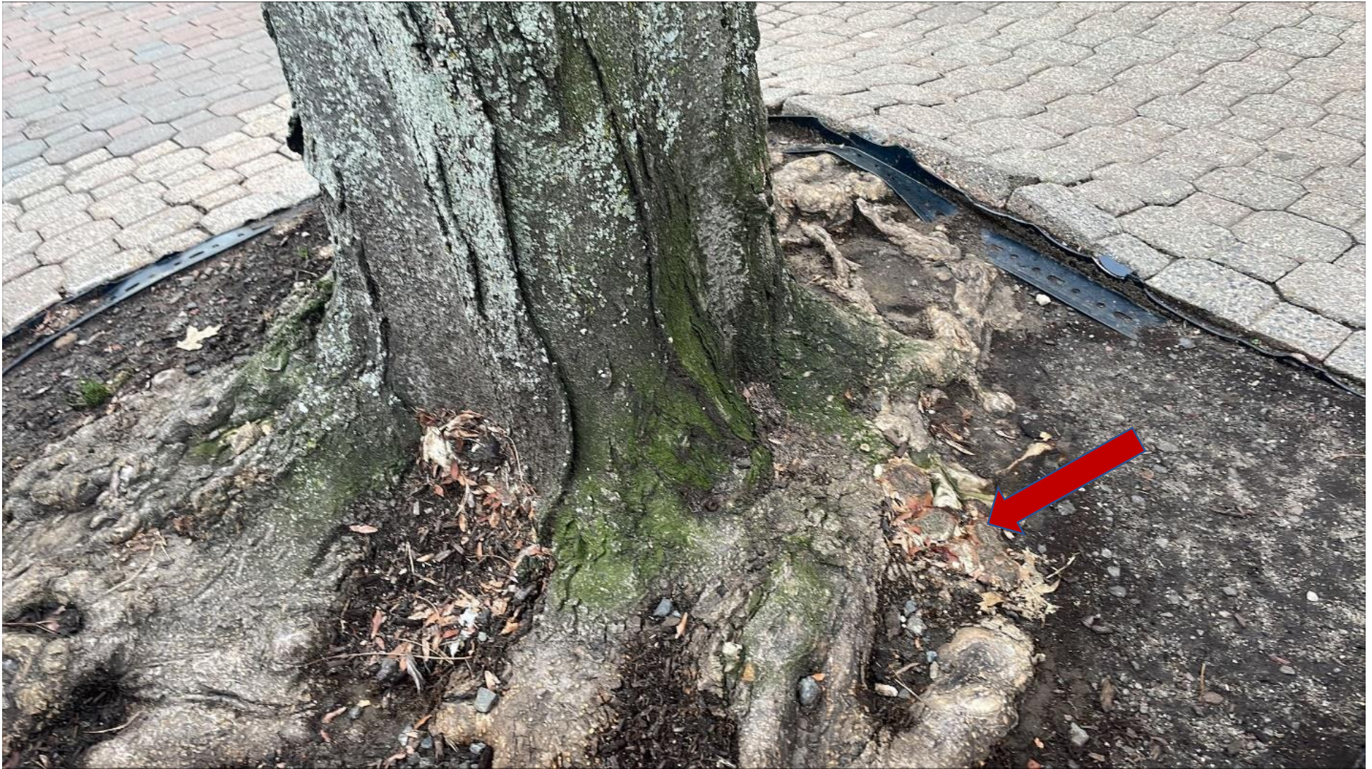
Thornless honey locust #81, showing damaged roots, sidewalk damage and fungal growth (arrow).
