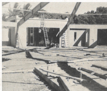
... and then we had walls and you could begin to see the shape of things to come.
