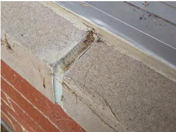
4. Some sealant shows early signs of deterioration.
