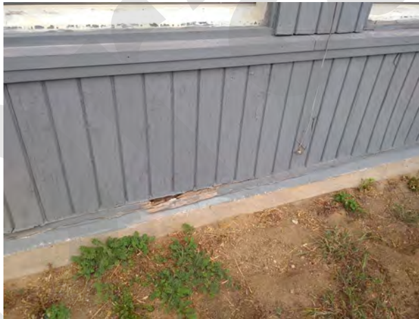
5. The wood siding is rotted and damaged.
