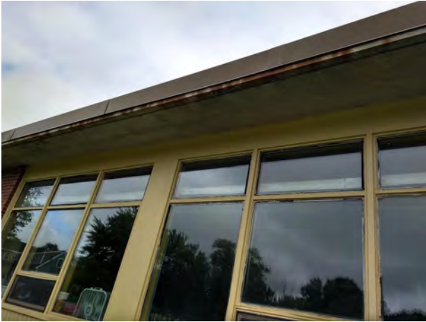
7. Original roof soffits have corroded.
