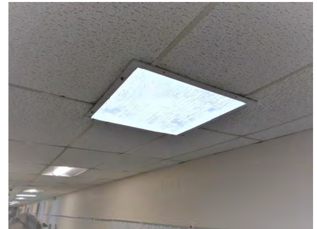
18. The skylights in the corridors are damaged.
