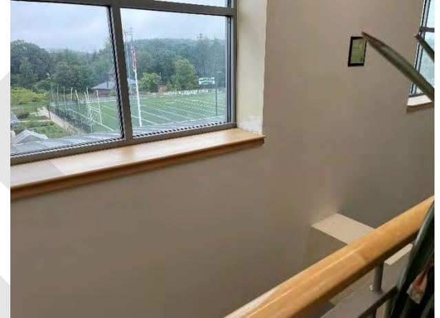
9. Several windows show signs of water damage.
