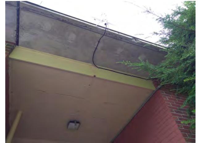
6. The concrete fascia and soffits have spalled.
