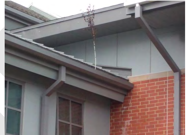
3. Some gutters are clogged with vegetation.
