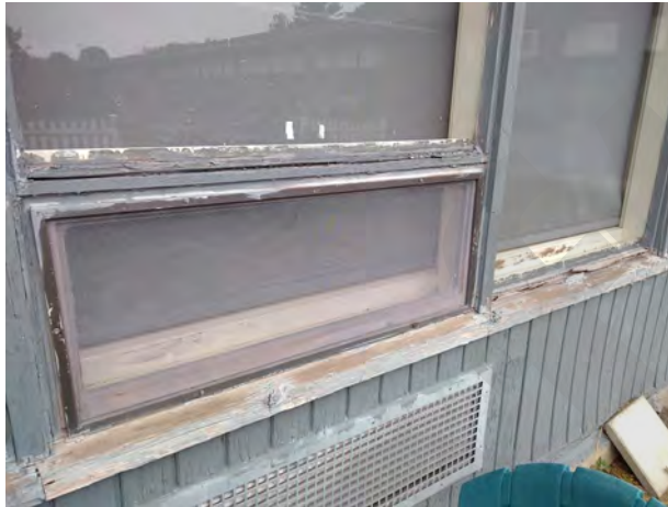
2. Original windows and trim have deteriorated.
