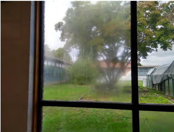
4. Thermal pane window has seal failure.
