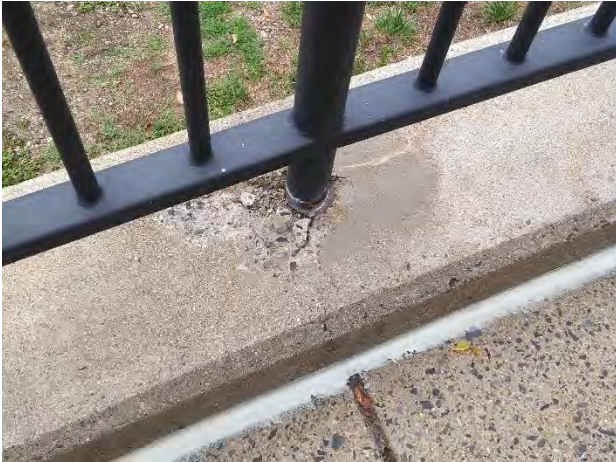
1. Concrete has spalled at some rail posts.
