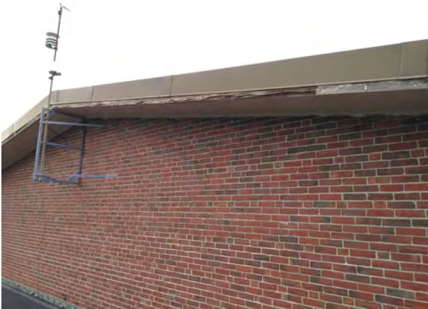
13. The fascia is rotted at the Cafetorium.
