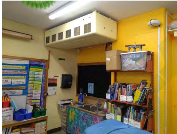
20. Classrooms have outdated and inefficient unit ventilators.
