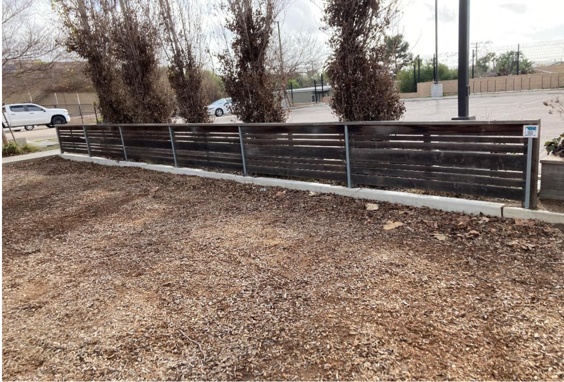
PHOTO 1 – Existing wood fence to be removed.
