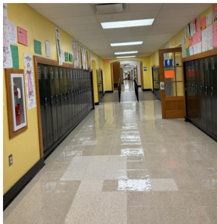
Flooring is aged and mismatching
