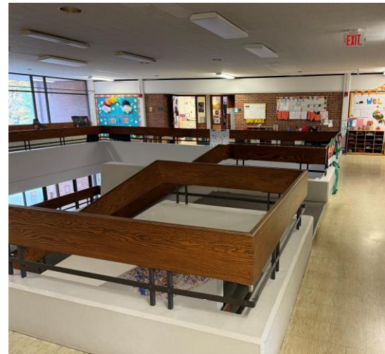
Guardrail height below Building Code
