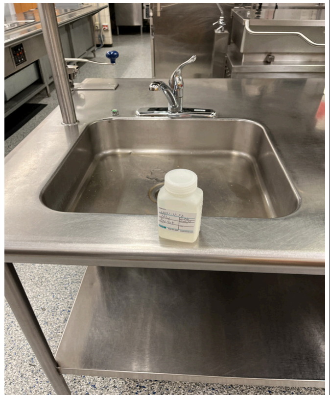
7/8/2024 - 13001-12 - Fleetridge Elementary - Prep Sink
