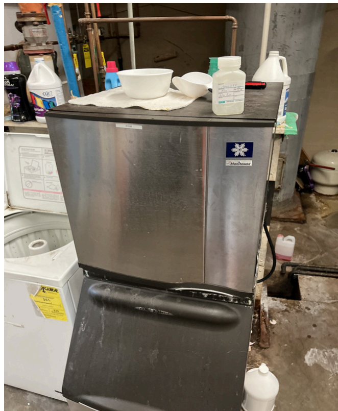
7/8/2024 - 13001-11 - Fleetridge Elementary - Boiler Room
