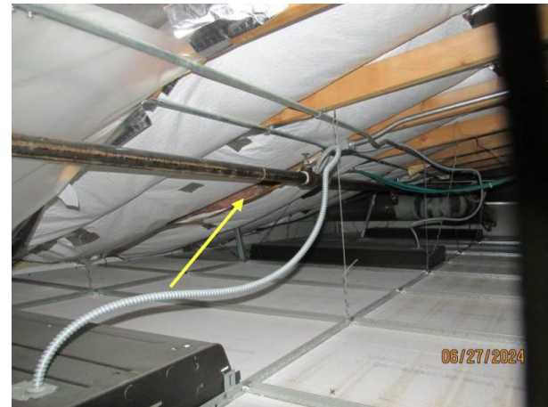
Open insulation gaps
