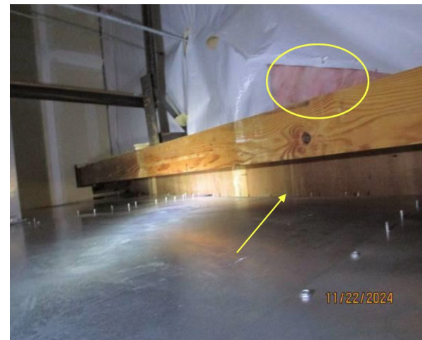
Vapor barrier gap and missing insulation
