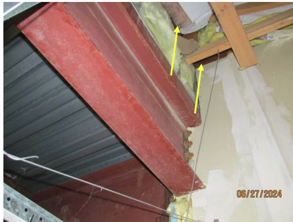
Open insulation gaps
