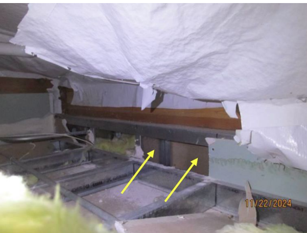
Missing batt insulation
