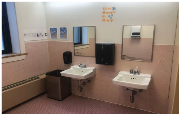
Non ADA Compliant Toilet Room
