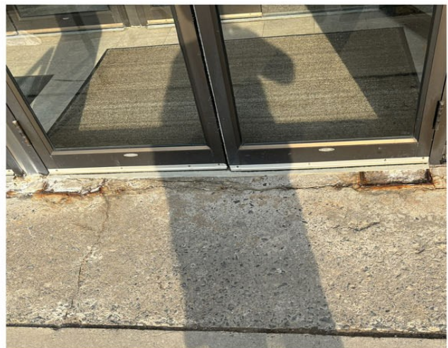
Deteriorated Stair Landing
