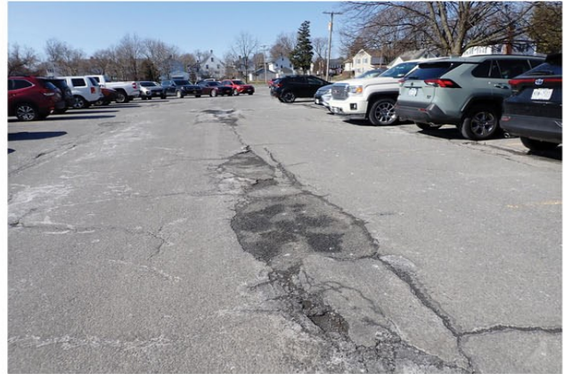
Deteriorated Parking Lot
