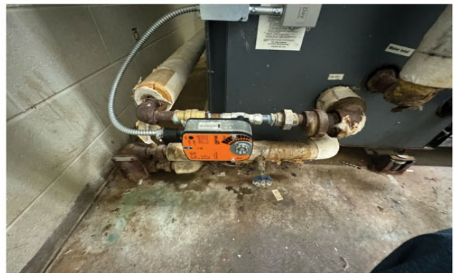
Failing Steam Control Valves to Hot Water
