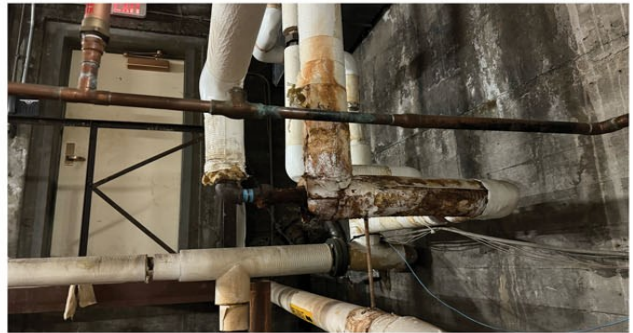
Failing Steam Pipes
