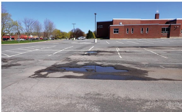
Deteriorated Parking Lot
