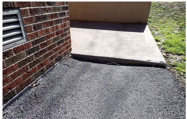
Non ADA Compliant Sidewalk
