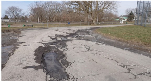
Failing Back Driveway
