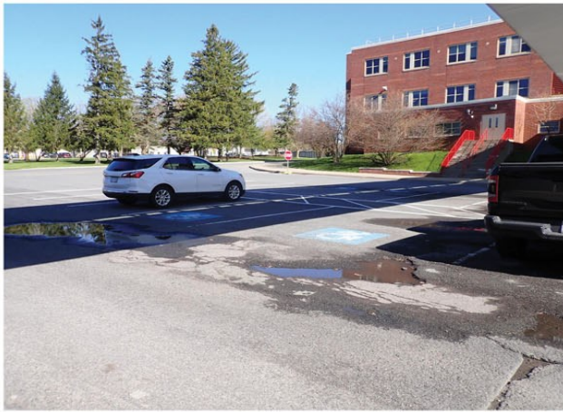
Deteriorated Parking Lot
