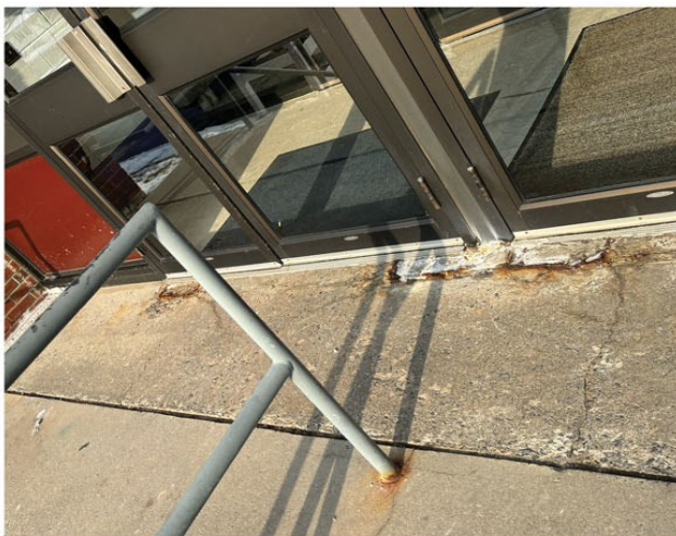
Deteriorated Exterior Doors
