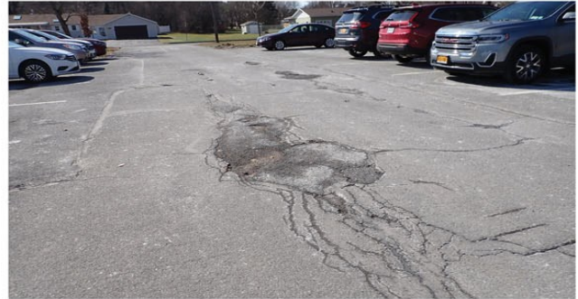
Deteriorated Parking Lot
