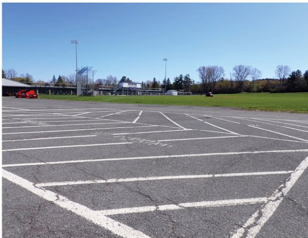
Deteriorated Parking Lot
