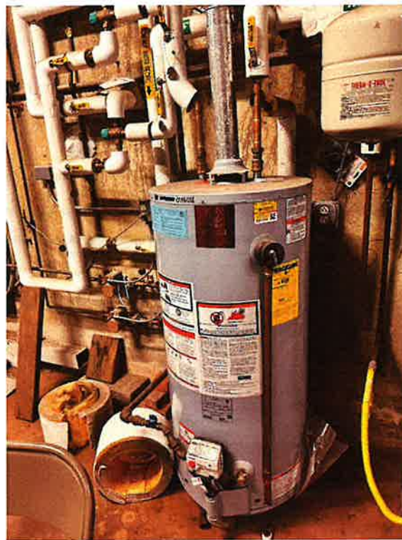
Photo 3: Domestic Hot Water Heater
