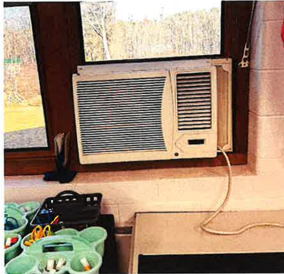
Photo 7: Window Air Conditioner
