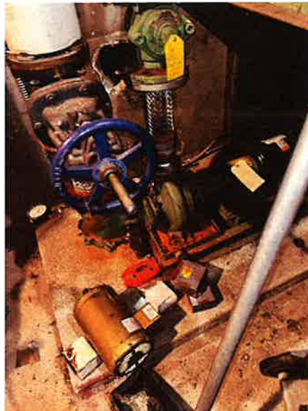
Photo 4: Hot Water Pump Condition
