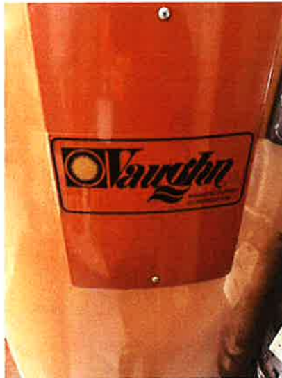
Photo 5: Domestic Hot Water Heater Condition
