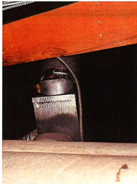
Photo 9: Attic Exhaust Fan
