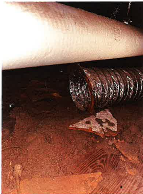
Photo 10: Attic Exhaust Fan
