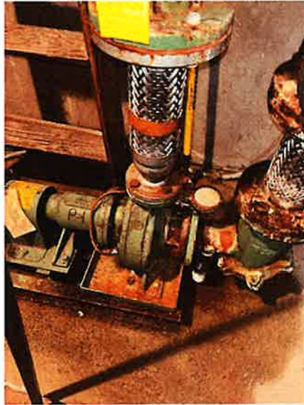
Photo 3: Hot Water Pump Condition
