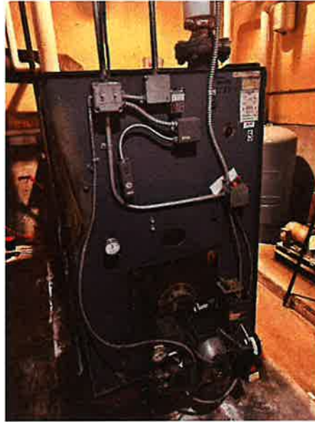
Photo 1: Hot Water Boiler
