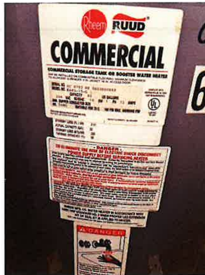
Photo 6: Domestic Hot Water Heater - Boiler Room
