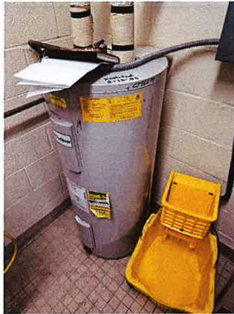
Photo 7: Other Hot Water Heaters
