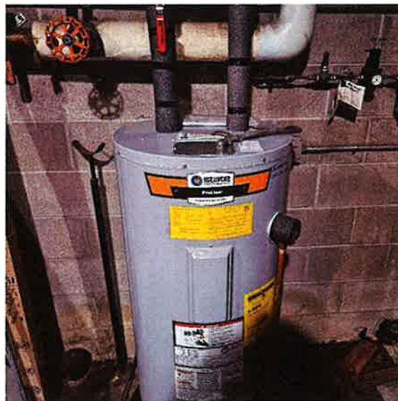
Photo 4: Domestic Hot Water Heater
