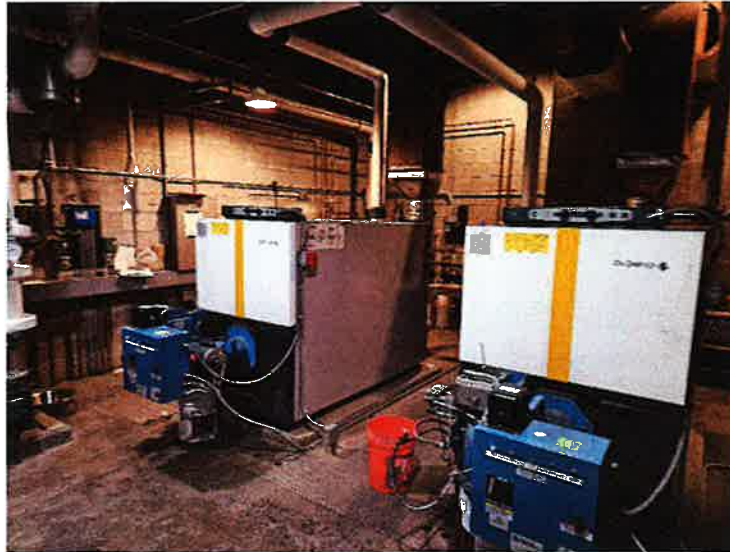
Photo 1: Hot Water Boilers
