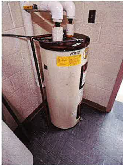
Photo 6: Other Hot Water Heaters
