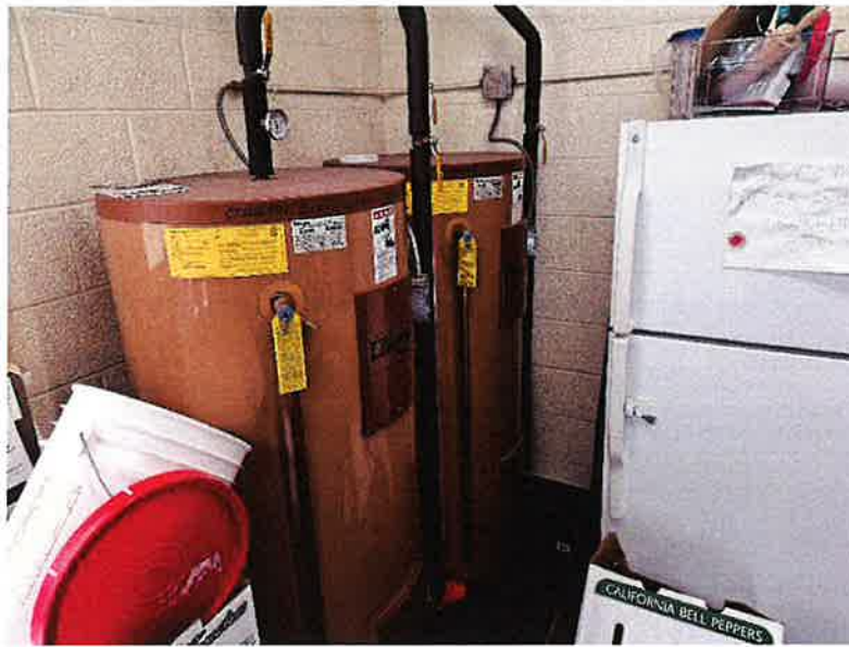
Photo 9: Other Hot Water Heaters
