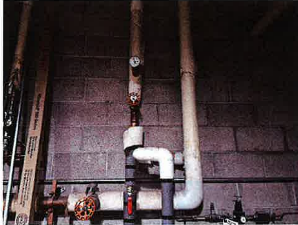
Photo 5: Domestic Hot Water Insulation
