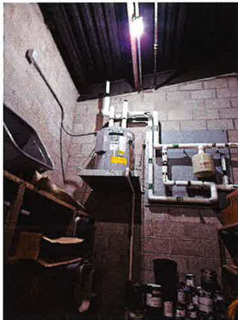
Photo 8: Other Hot Water Heaters
