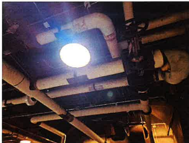
Photo 2: Hot Water Piping
