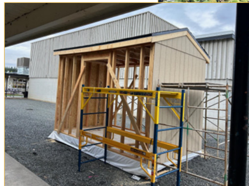
Below, one of the Project Hope sheds being assembled in the workyard.
