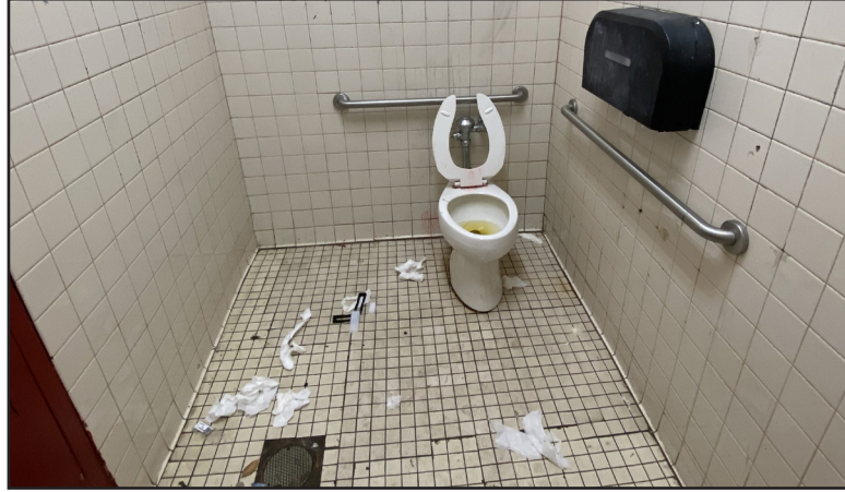
Would you want to use this bathroom? With toilet paper strewn on the floor and urine in the toilet, custodians are the people cleaning up this mess.
