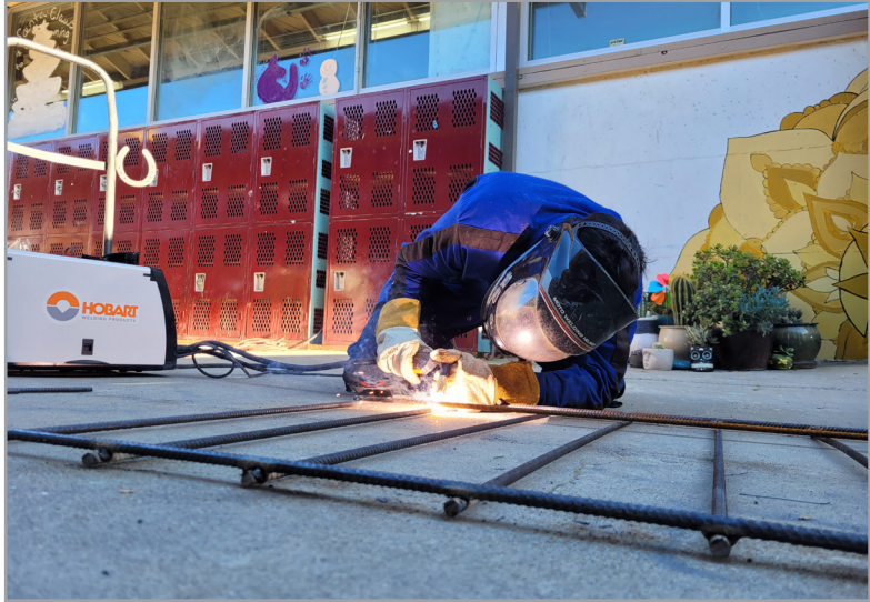
Diego Lopez demonstrates his newly-learned skill of welding to build the base of the project. Photo by Kristiana Zaste
