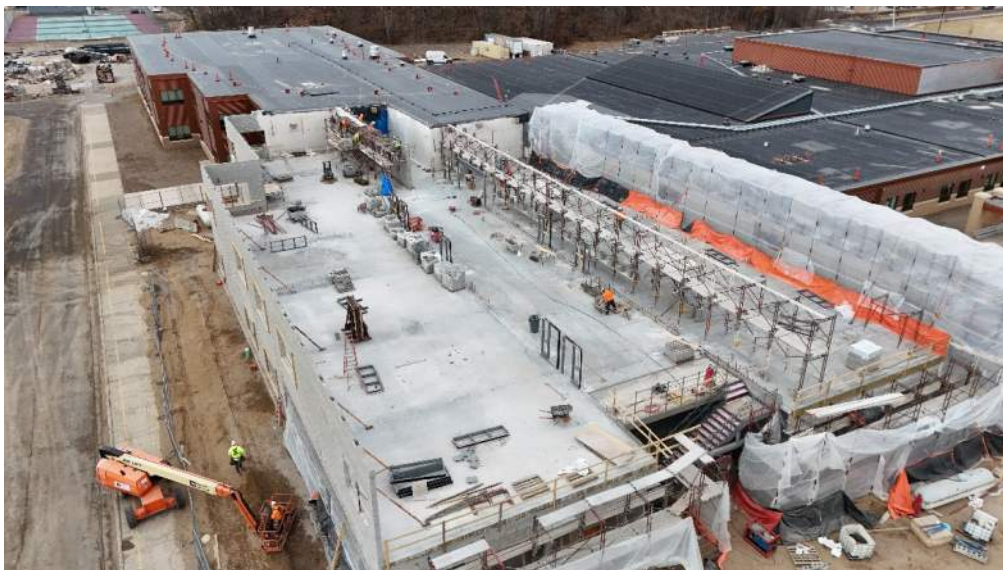
Aerial View - Segment H Classroom Addition 2 nd Level CMU Exterior Bearing Walls
