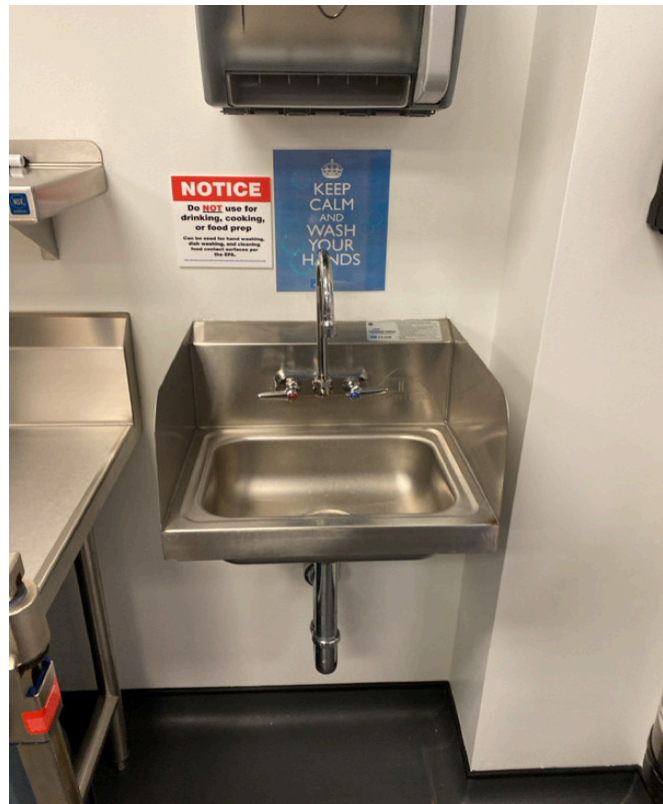
4/19/2024 - 6889-23 - NIC - Kitchen-Southwest Handwashing
