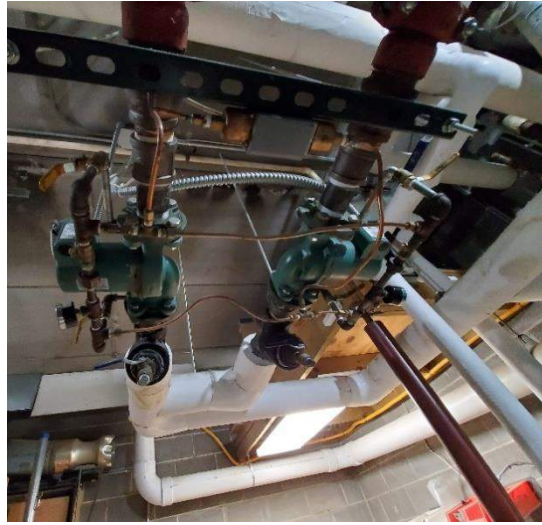
Photo 2: Hot water pumps
