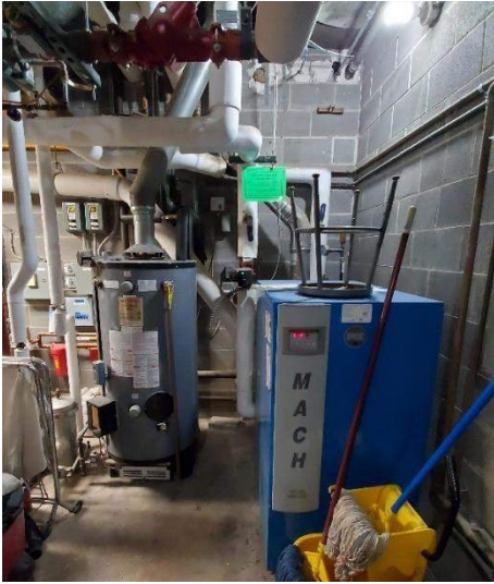
Photo 1: Water heater and boiler
