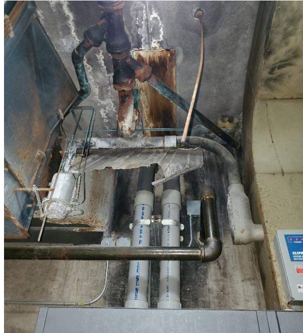
Photo 2: West Elementary drain above electrical service
