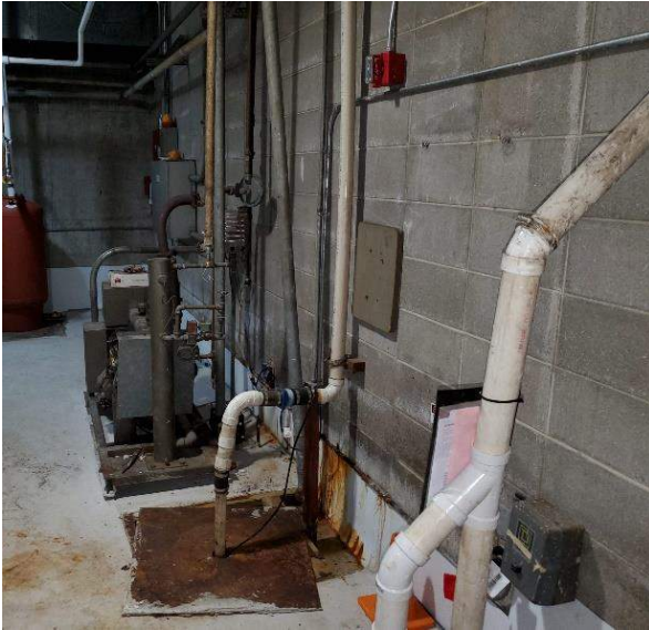
Photo 1: West Elementary sump pump
