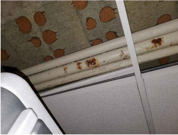
Photo 1: Corroding sanitary drain piping
