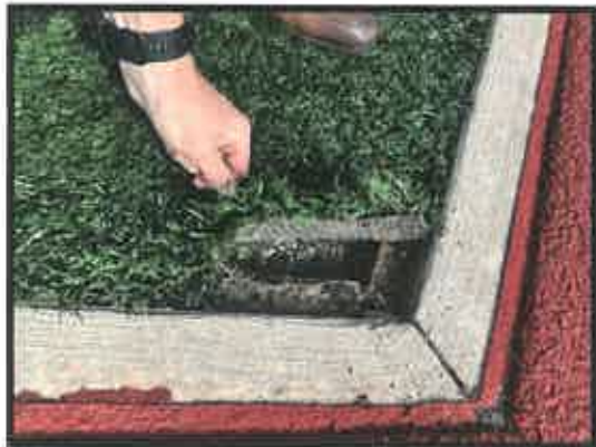
Settlement along track edge
