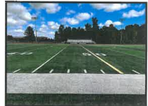
Visible seams that have raised / opened
