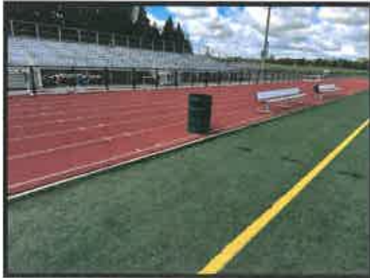
Settlement along track edge
