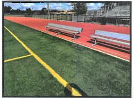
Damage & settlement at utility box
