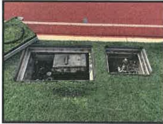
Damage & settlement at utility box
