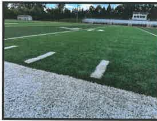
Visible seams that have raised / opened
