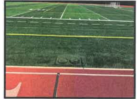
Damage & settlement at utility box
