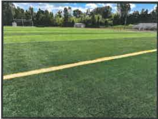
Visible seams that have raised / opened & wrinkle at 50 yardline
