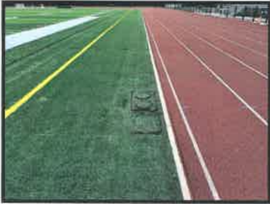
Damage & settlement at utility box
