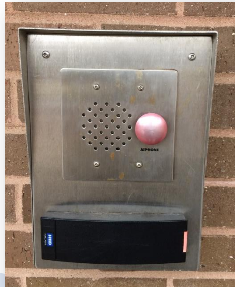
Visitor Entrance Intercom to front office
