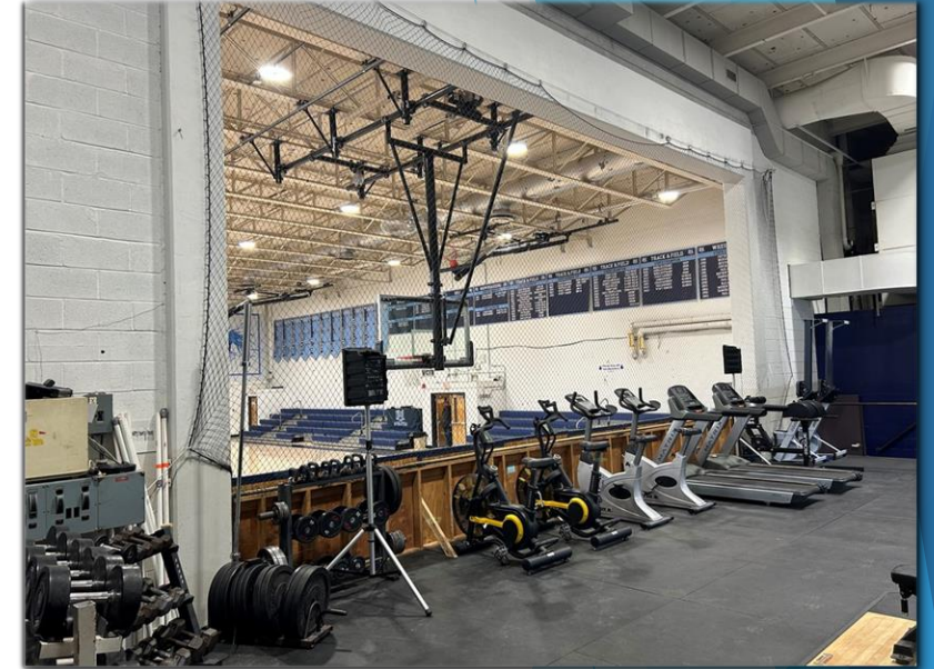
Exposed combustible framing at former RUHS gym stage proscenium opening. Combustible framing materials are not permitted in construction type. Combustible framing and materials have been observed in numerous areas throughout RUHS/RUMS/RTCC
