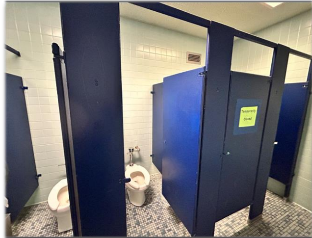
141 Bathroom - Non-ADA, old fixtures & partitions, old floor & wall tile finishes. Recurrent concerns through Middle/High School & Brookfield Elem. with minimal ADA access bathrooms
