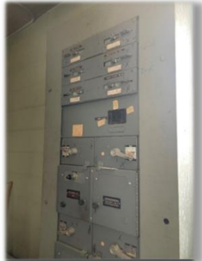
Very old 480-volt fused switch panelboard
