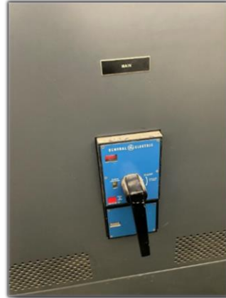
Switchboard protection device with no ground fault protection or energy reduction switch (ERMS)
