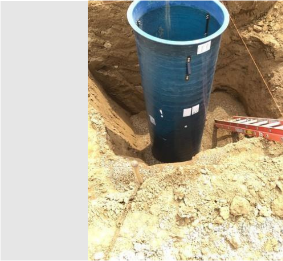
Description: Crock for elevator sump
